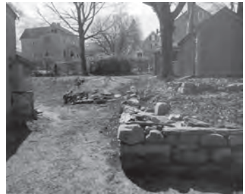
After all the ivy was removed and repairs made, we have beautiful stone garden walls!
