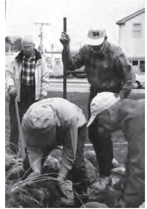
Our president, Brad Gorham, center, helped to repair the wall back in 2001, along with Harold Ordway, Tom Hall and Victor Fox.
